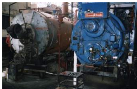
Figure 4-20: Fuel oil operated boilers [87]
