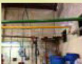
Steam system measures
